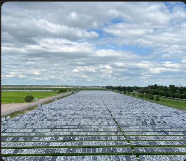
Example of a solar farm damaged by hail, Nebraska 2023 • Nebraska Public Power District
