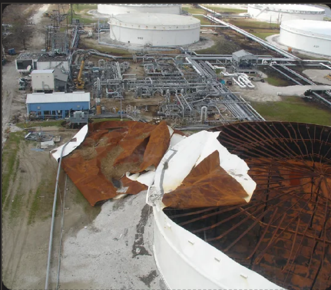
Example of a storage tank that experienced wind damage
